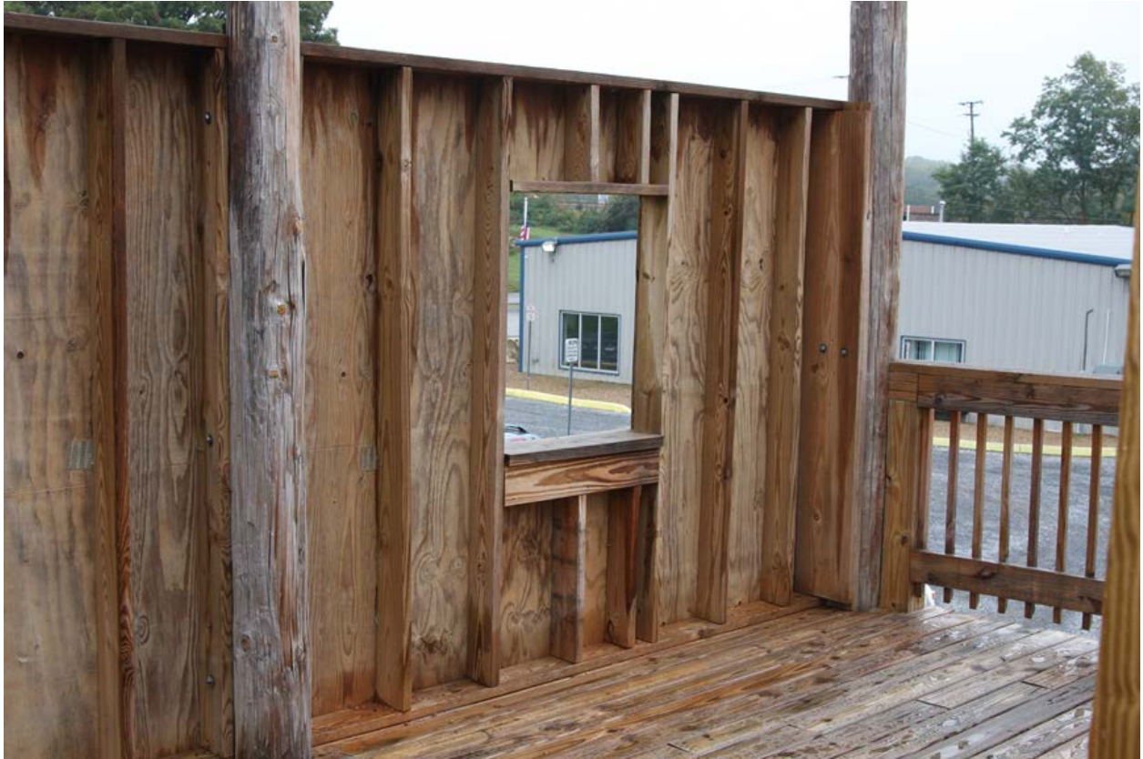
The second floor of wooden drill tower showing the window opening for ladder placement evolutions and the floored work area of adequate size for firefighters to stand and work.
