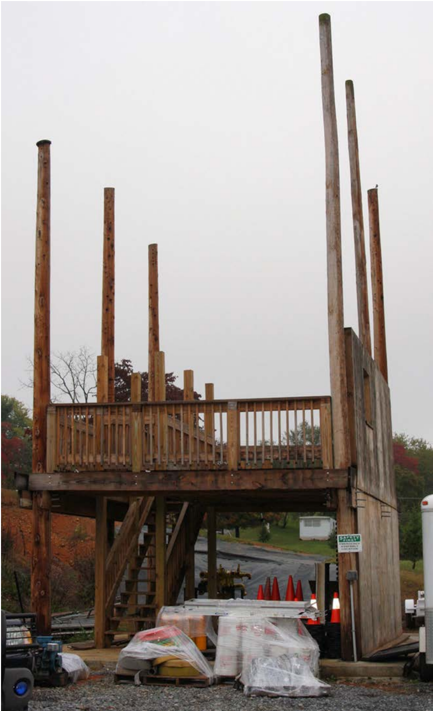
Three story drill tower under construction in Mt. Carmel, Tennessee. Built-in stairs allow hose advancement drills and easy access to the upper floors.
