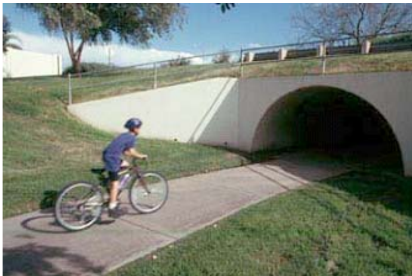
Figure 19. Grade-Separated Crossing (Tunnel) Under a Roadway. From www.pedbikeimages.org/ Dan Burden. Reprinted with permission.
