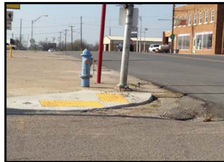
Non-Flush Curb Ramp Transition
