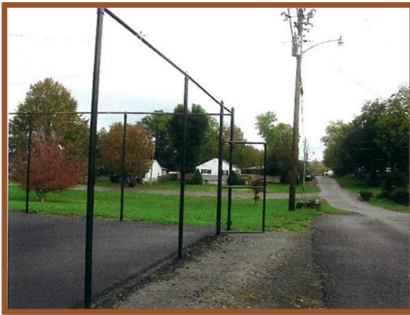
Fifth and Filbert Park missing fence
