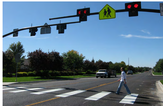
High-Intensity Pedestrian Activated Crosswalk and Signal
